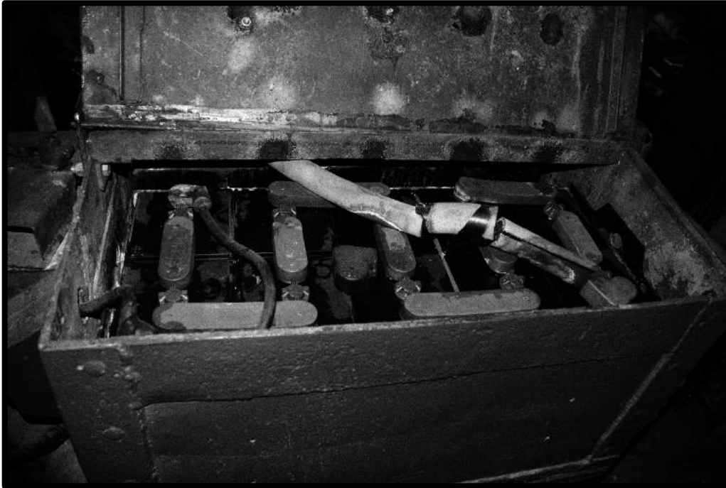
Batteries inside a Mancha Locomotive ( see p. 86, paragraph 6 & p.89, para. 2)
