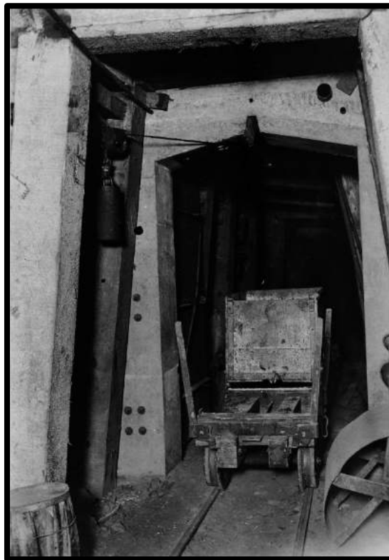
Concrete and steel fire doors near a shaft. The two mine cars blocking the doors were a safety concern. The doors would be blocked from shutting. (see p.32, para. 4)
