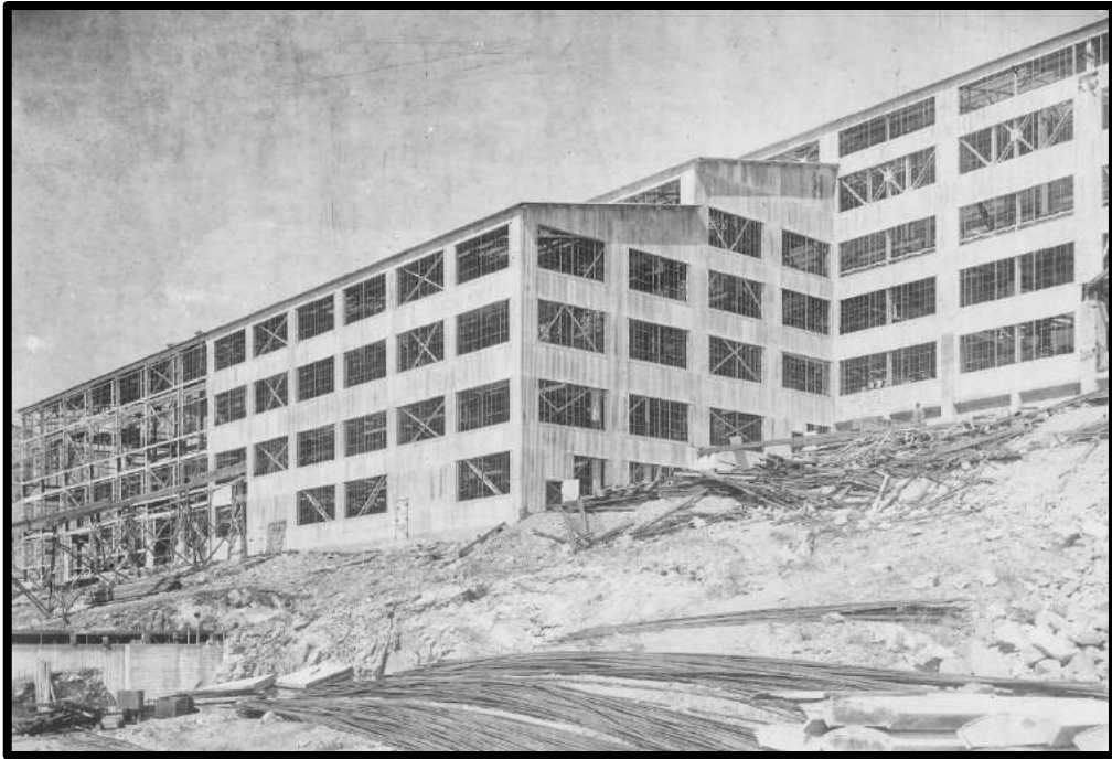
Two views of construction on the Sacramento Concentrator in 1921 (see p. 45, para. 6)
