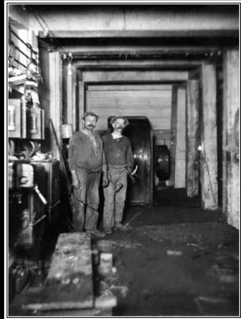
GRAEME LARKIN COLLECTION INSTALLING A LARGE VENTILATION BLOWER IN THE GARDNER MINE - 1912
