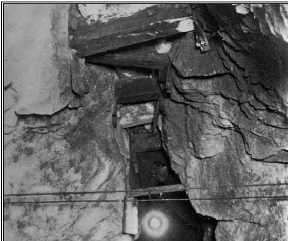
Fissure on the 200 level, Czar Mine (Douglas, 1900). This was undoubtedly a subsidence caused, marginal crack.
