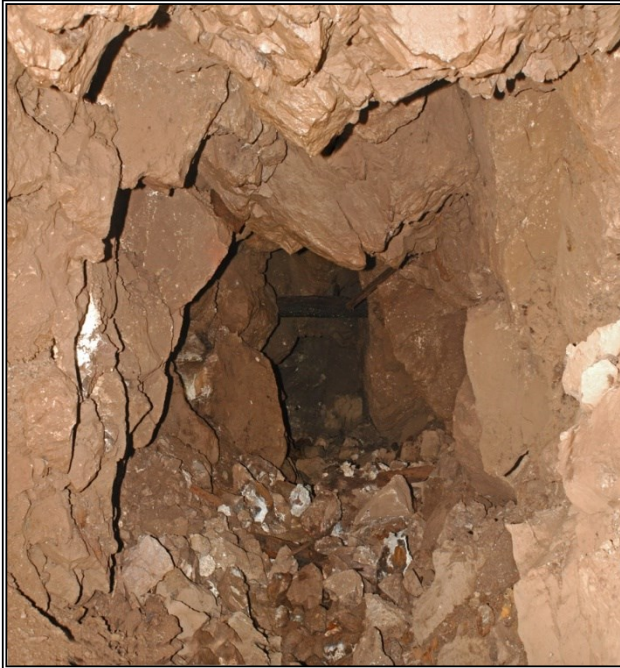
A crosscut driven through blocky, chaotic boulders of broken limestone showing dilation and breakage along bedding planes, subsequently cemented by minor calcite. A feature such as this was an important guide to possible ore somewhere below. This is 86 Crosscut on the 6 th level of the Southwest Mine and mining through this broken rock would have been both difficult and dangerous as large blocks of limestone fell from the sides and back (top). Maximum width - 3.5 meters. Graeme/Larkin collection.
