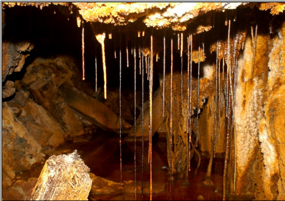
Acidic mine water formed by the oxidation of pyrite. Mud-like iron hydroxides have precipitated from the water and partially filled the mine opening. Tan colored melanterite locally coats the mine walls. 7 th level, Southwest Mine, horizontal view – 2.2 meters. Graeme/Larkin collection.
