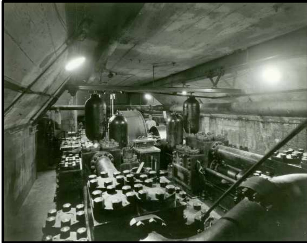
Pumps at the 2200 level Junction Mine
