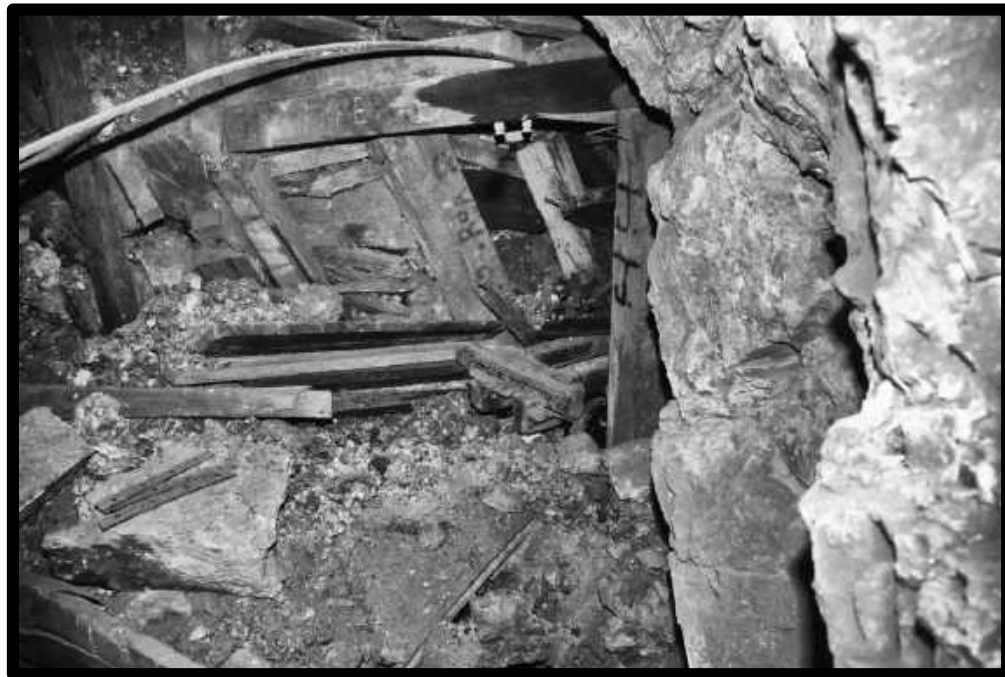
The collapsed B level station of the Copper Queen Mine
