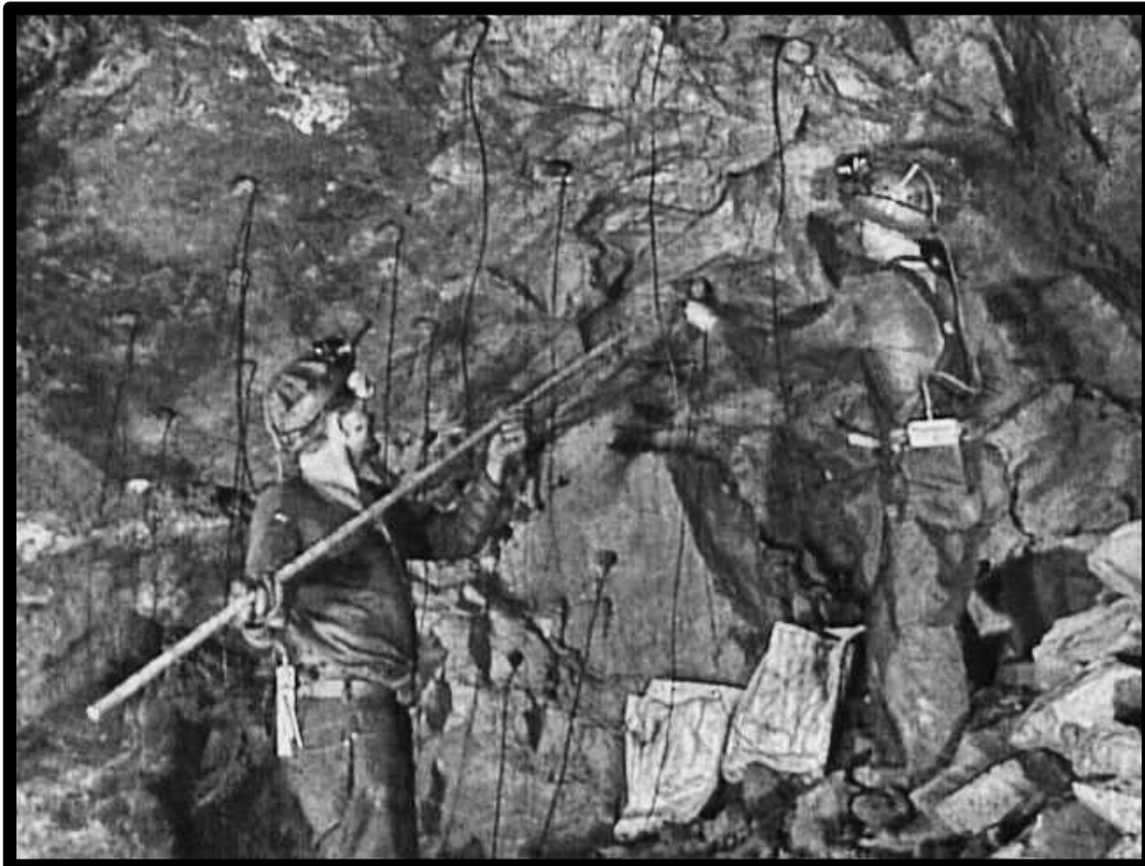
Loading blast holes in an Incline Cut & Fill Stope, Campbell Mine, c-1940
