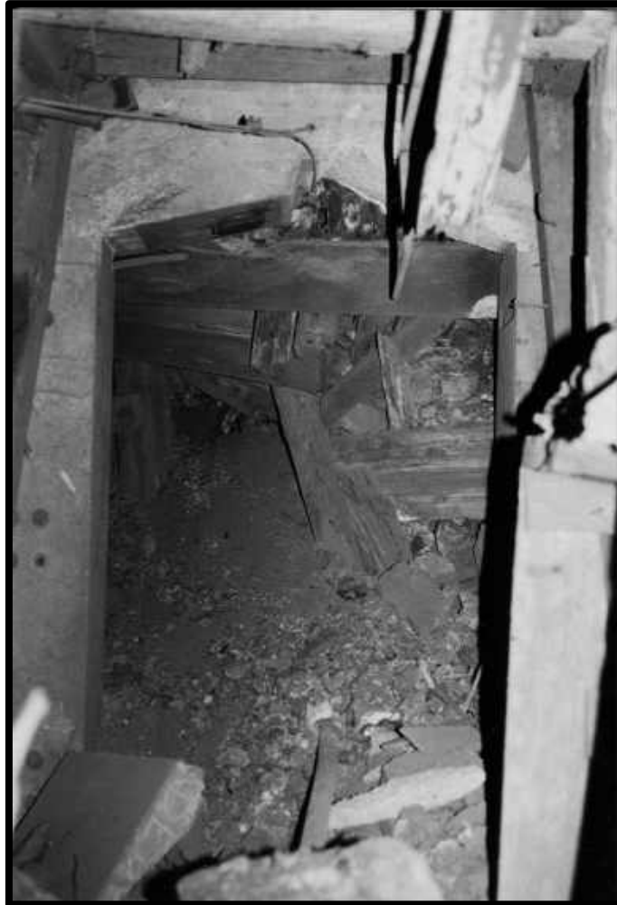
A caved-in crosscut just off the 3 rd level of the Southwest No.3 Shaft station. Note, the concrete frames of the fire door.
