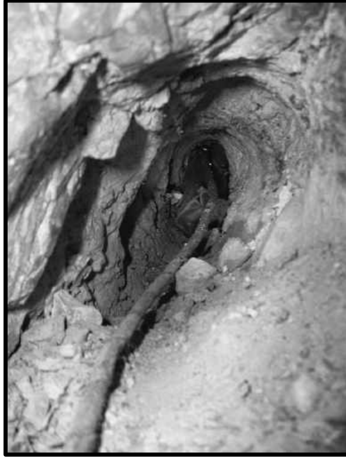
View into a misfired hole revealing a stick of dynamite and a fuse. This image was taken in the Georgia Tunnel.
