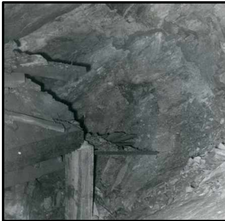
A view of the source of the caved rock from the previous picture (top center.) The point of the gin pole seen in the previous picture is located just above the standing square set post. 31-B stope 3100 level.
