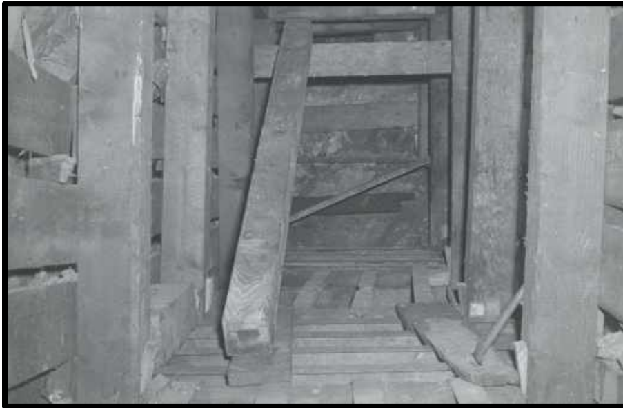
A fallen stringer at the top of grizzlies in a stope. This is the location B.W. Childress was injured. 2400 level Junction
