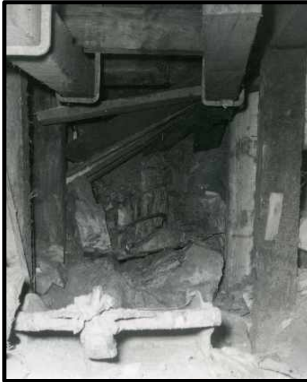
A view of the caved face in 31-B stope on the 3100 level. This is the site H. Orton was injured. In the foreground is a slusher rake. At the center and just above the end of the scaling bar is the head to Orton's wheat lamp among the fallen boulders. Hidden in the left corner is a gin pole with a paper tag hanging from it
