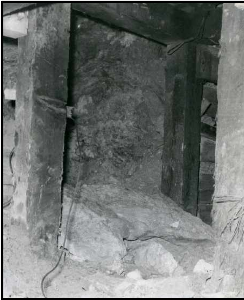
The boulder that killed F.R. Burgos lying on the ground. 143 crosscut 2700 level Campbell Mine
