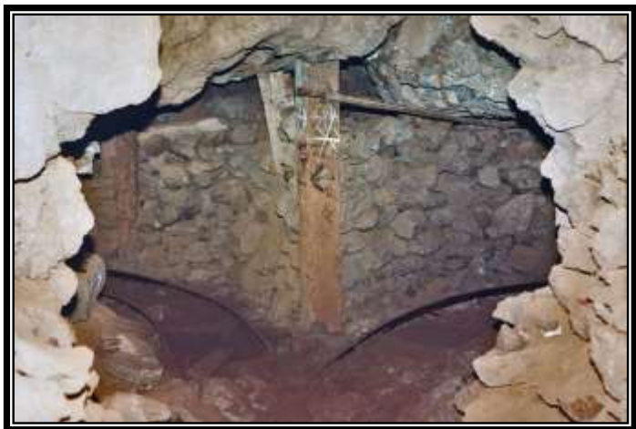
Gob walls made from waste manually sorted from ore in a stope, 5 th level Southwest Mine Graeme Larkin collection
