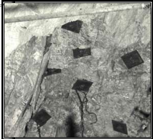
Expansion shell, rock bolts in place 3100 level Denn mine Graeme Larkin collection
