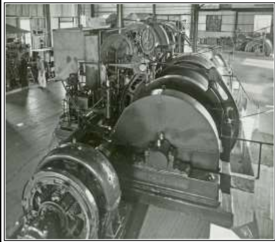
VIEW IN THE JUNCTION HOIST HOUSE - 1934, WITH THE MAN HOIST (1 & 2) IN THE FOREGROUND, SKIP HOIST (3 & 4) IN THE MIDDLE GROUND AND THE SERVICE HOIST (5) IN THE FAR RIGHT
