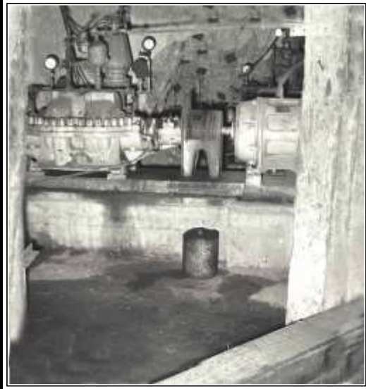
GRAEME LARKIN COLLECTION ONE OF THE PUMPS ON THE 3100 LEVEL DENN MINE -1962
