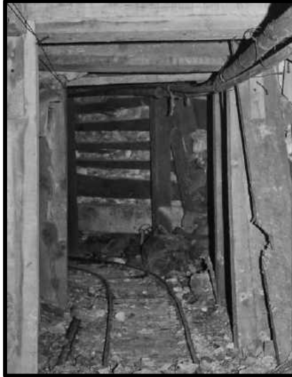
SPLIT LAGGING ON THE 1 ST LEVEL OF THE HARGIS INCLINE.
