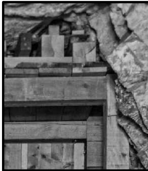
Block(s)(DEF. 1) SECURING A DRIFT SET TO THE BACK (CEILING) OF 30 CROSSCUT, 3 RD LEVEL SOUTHWEST MINE.
