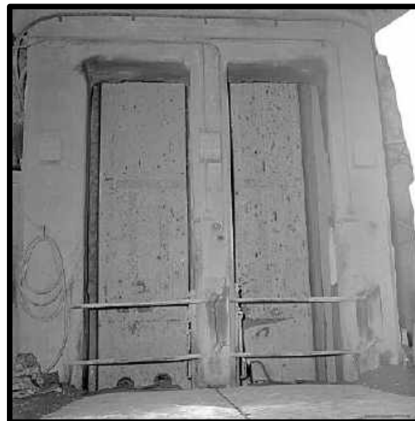
SHAFT DIVIDER MADE OF CONCRETE AT THE 2966 LEVEL OF THE CAMPBELL MINE.
