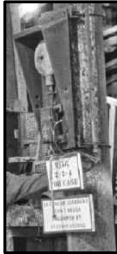
CALL BELL, 2700 LEVEL, STATION, JUNCTION MINE
