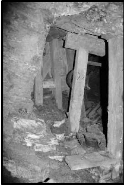
T STALL IN THE STOPPED OUT 45 CROSSCUT ON THE 6 TH LEVEL OF THE SOUTHWEST MINE.
