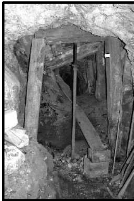
CATCH UP GROUND A TIMBER JACK INSTALLED AS MINERS ARE TRYING TO SUPPORT A CAVING CHUTE IN 61 CROSSCUT ON THE 3 RD LEVEL OF THE SOUTHWEST MINE.
