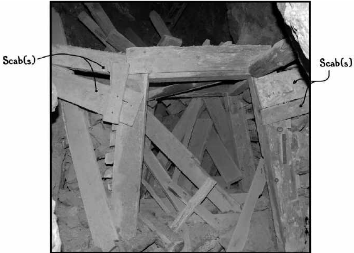
SCAB(S) (DEF.2) ON A DRIFT SET IN 35 CROSSCUT 5 TH LEVEL SOUTHWEST MINE
