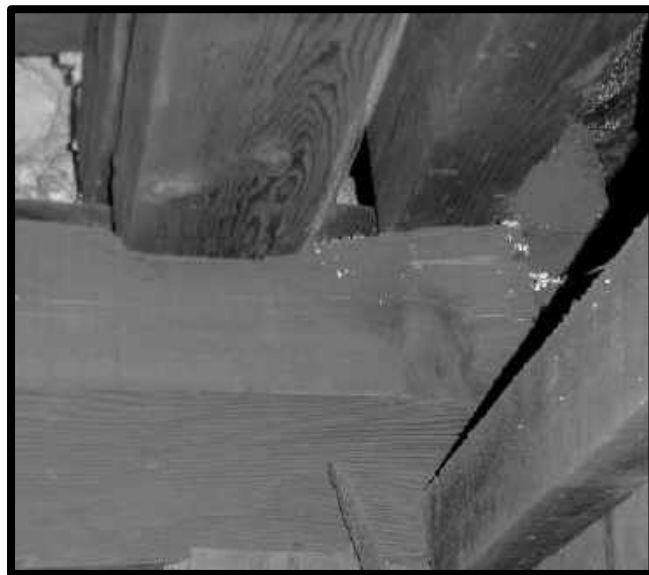
TAKING WEIGHT BLOCKS BEING CRUSHED ABOVE A CAP AT THE 3 RD LEVEL SOUTHWEST SHAFT STATION
