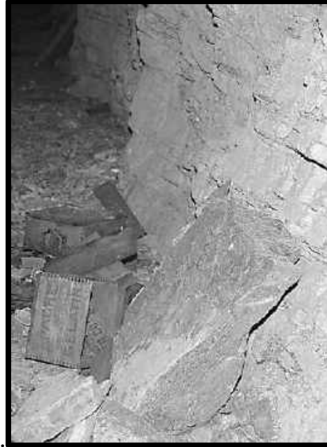
SLAB THAT HAS FALLEN IN AN ABANDONED POWDER MAGAZINE IN 10 CROSSCUT, 6 TH LEVEL SOUTHWEST MINE
