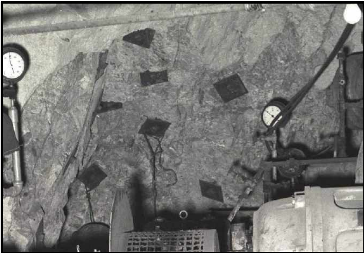
TIE PLATE(S) (DEF. 1) ON ROCK BOLTS AT THE 3100 LEVEL PUMP STATION DENN MINE.
