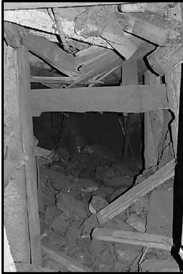
SAGGING GROUND 3 CROSSCUT 3 RD LEVEL SOUTHWEST MINE THE TIMBER IS BEGINNING TO SAG
