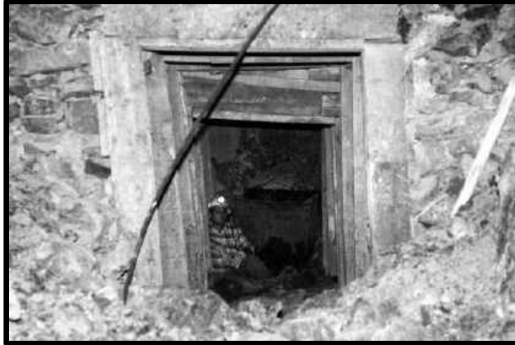
HEAVING IN A SUBLEVEL CROSSCUT IN THE WOLVERINE COUNTRY OF THE HIGGINS MINE. THE FLOOR HAS BEEN RAISED AT LEAST 16 INCHES FROM HEAVING
