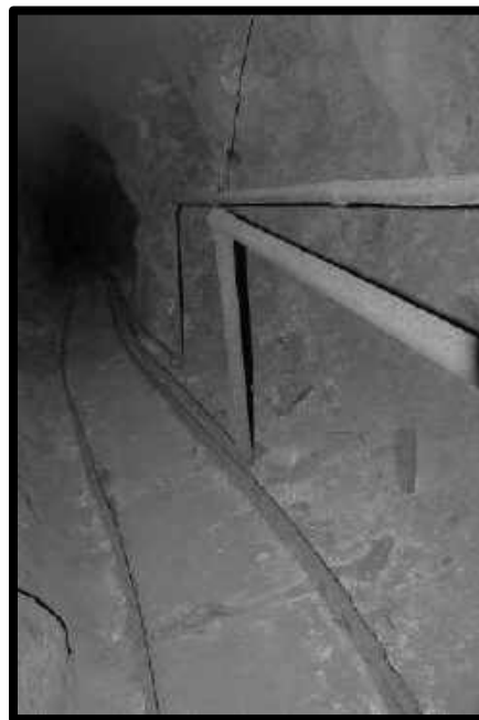
AIR LINE IS THE LOWER PIPE WITH THE WATERLINE ABOVE. SOUTHWEST MINE, 4 TH LEVEL
