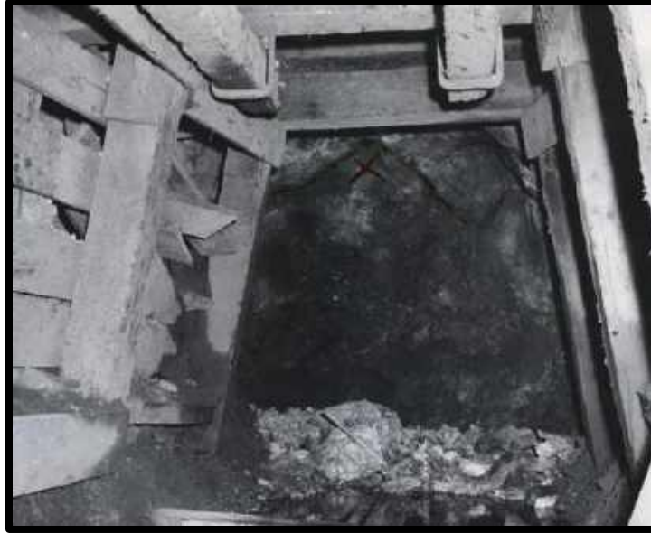
FALL OF GROUND IN 22 CROSSCUT ON THE 2966 LEVEL, CAMPBELL MINE
