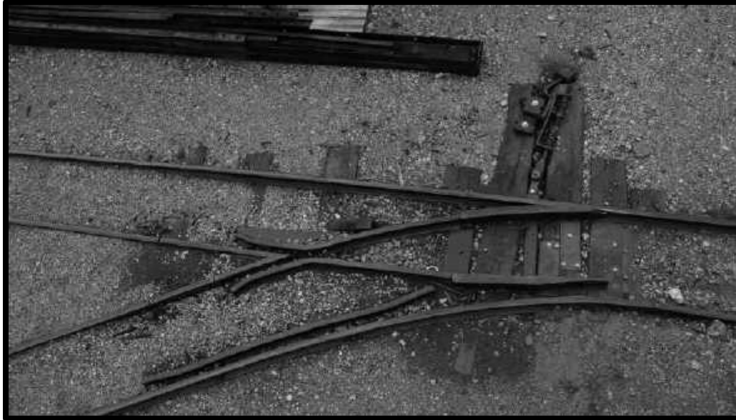
SWITCH (DEF. 1) LOCATED AT QUEEN TUNNEL PORTAL
