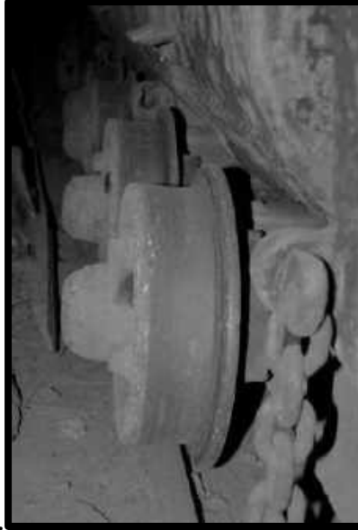
FLANGE (DEF. 1) ON A H-CAR WHEEL ON THE 3 RD LEVEL OF THE SOUTHWEST MINE
