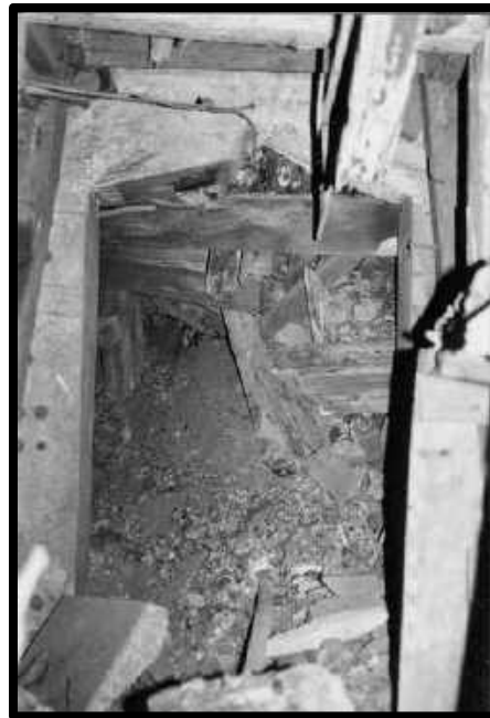
CAVE-IN RIGHT AT A FIRE DOOR IN 3 CROSSCUT ON THE 3 RD LEVEL SOUTHWEST MINE.
