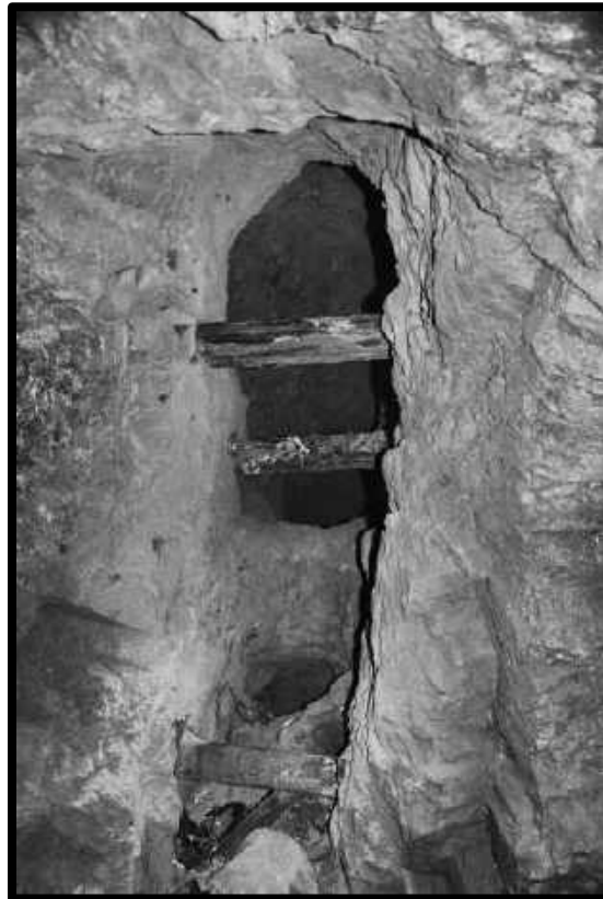
STULL(S) IN A NARROW STOPE ABOUT 3 1/2- 4 FT. WIDE, 6 TH LEVEL SOUTHWEST MINE
