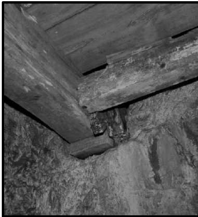
HITCH CUT TO SUPPORT A BULKHEAD IN 30 CROSSCUT, 3 RD LEVEL SOUTHWEST MINE
