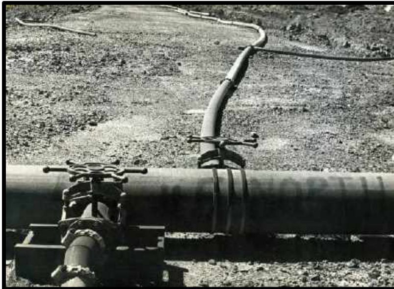
LEACH LINES ON #7 DUMP
