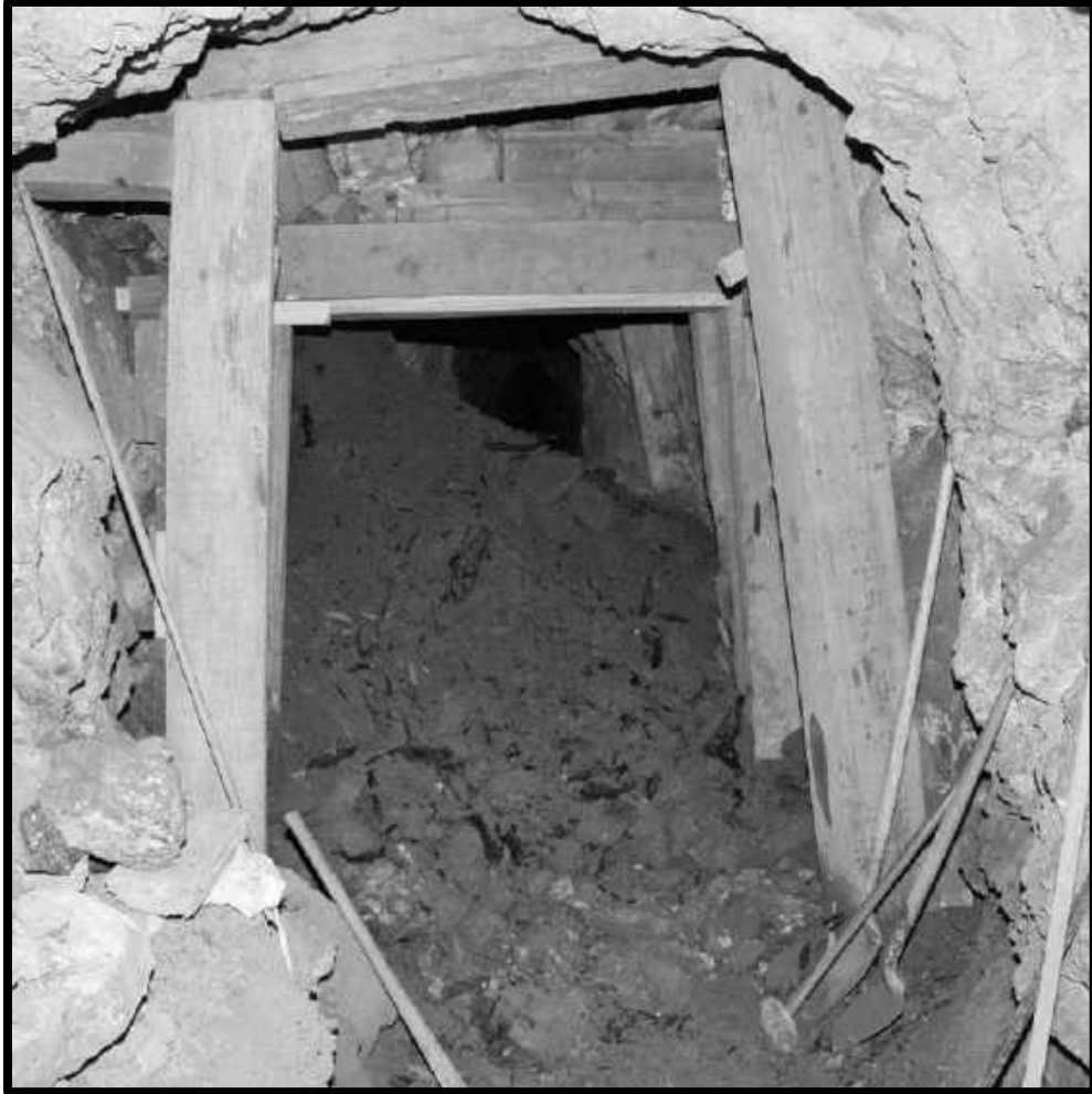
MUCK SPILLED FROM A CAVED, 33-1 CHUTE IN 61 CROSSCUT, 3 RD LEVEL SOUTHWEST MINE
