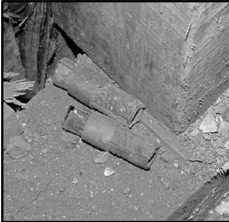
ROOF BOLT SHELL(S) 61 CROSSCUT, 3 RD LEVEL SOUTHWEST MINE
