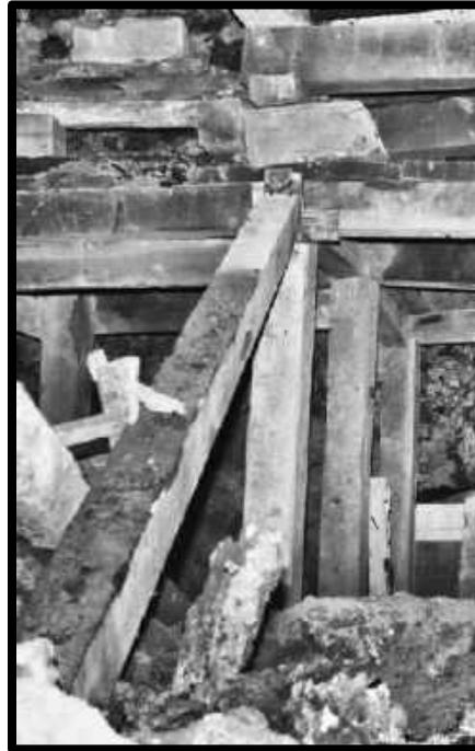
KNEE BRACE SECURING SQUARE SETS IN THE WOLVERINE COUNTRY OF THE 7 TH LEVEL OF THE SOUTHWEST MINE
