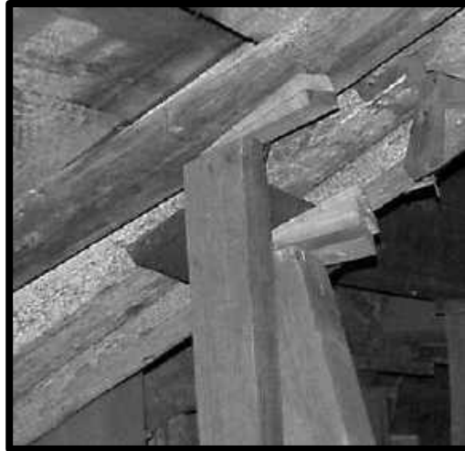
WEDGE(S) SECURING SPRAGS 3 RD LEVEL SOUTHWEST SHAFT STATION
