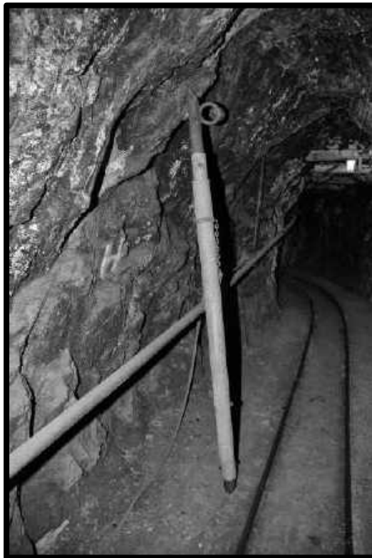
GIN POLE (DEF. 1) SOUTHWEST MINE, 3 RD LEVEL, 30 CROSSCUT.
