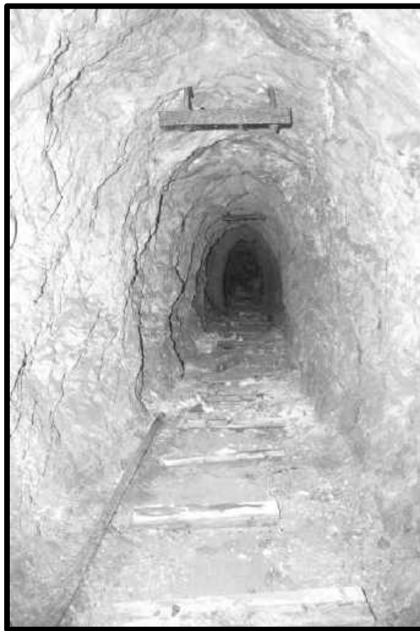
DEAD WORKINGS 43 CROSSCUT 3 RD LEVEL SOUTHWEST MINE. THE CROSSCUT WAS STRIPPED OF TROLLEY WIRE, RAIL AND AIR AND WATER LINES THEN ABANDONED LEVEL A DAMAGE SECTION OF PIPE AND OLD TRACK TIES REMAINING
