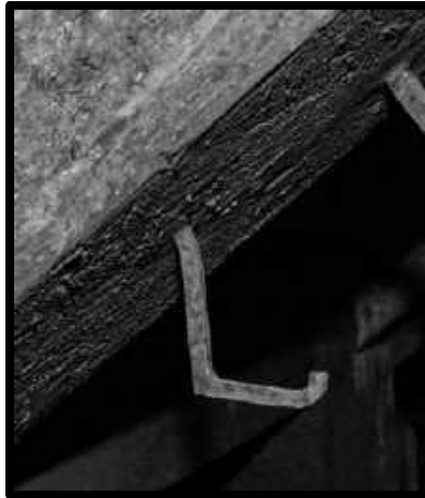
LADDER HANGER 3 RD LEVEL SOUTHWEST STATION, BENT SLIGHTLY OUT OF ITS ORIGINAL SHAPE
