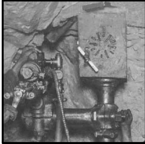
HEADBLOCK ON TOP OF COLUMN C-1903. NOTE THE STAR-LIKE PATTERN LEFT BY THE IMPRESSION OF THE TOP OF THE COLUMN BY A PREVIOUS USE.
