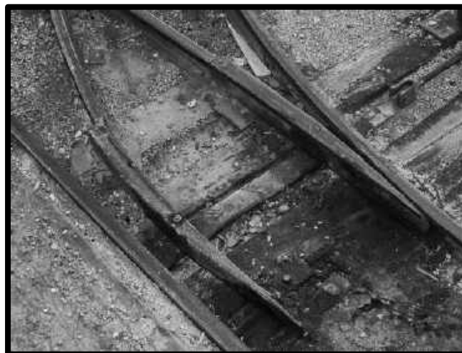
SWITCH POINT(S) AT THE QUEEN TUNNEL PORTAL.
