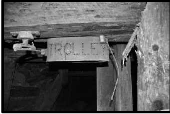
BLOCK LIGHT , AN EARLY STYLE ON THE SOUTHWEST SHAFT, 3 RD LEVEL STATION.
