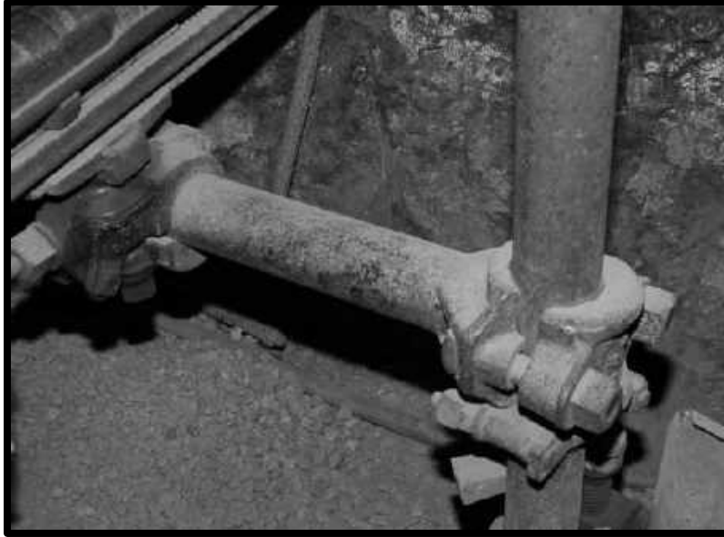
BAR (DEF.2) ON A COLUMN SOUTHWEST SHAFT, 3 RD LEVEL, STATION
