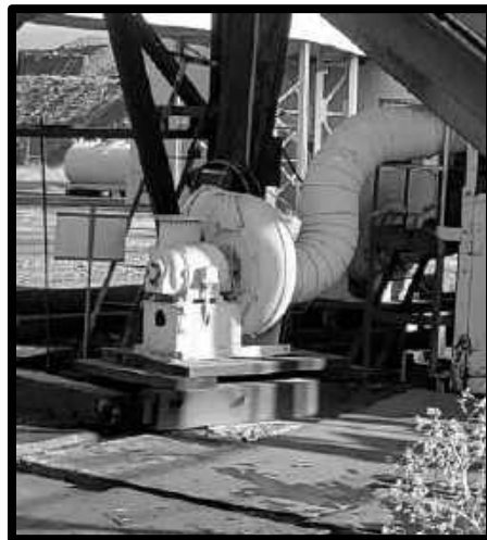
BLOWER AT THE COLLAR OF THE JUNCTION SHAFT. NOTE THAT IS BEING USED AS A SUCTION FAN DRAWING AIR OUT OF THE SHAFT.
