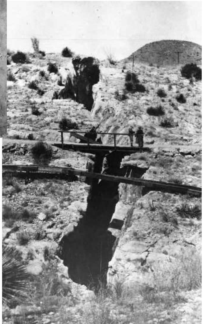
Figure 2.1.4: Subsidence crack with substantial displacement showing horizontal movement. By 1930 the crack had widened to the point that the bridge fell in to it. This was located to the south of the Holbrook Mine, 1913.
