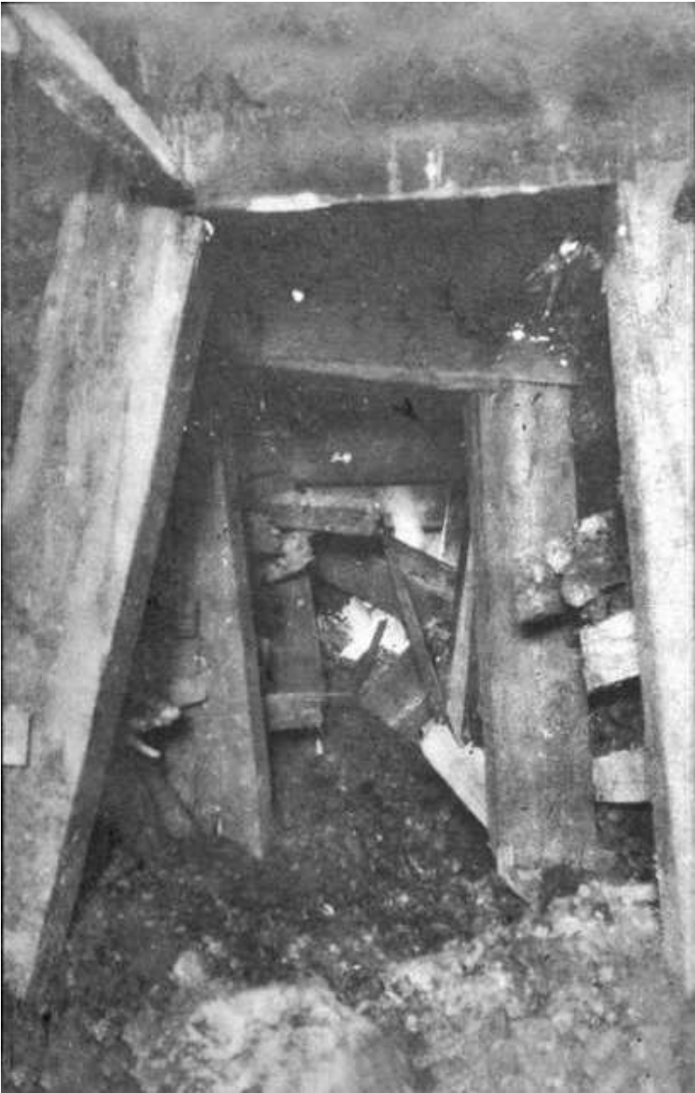
Figure 2.1.2: Typical collapse of mine workings caused by the crushing pressure of the ever-moving claylike ground in the Czar-Holbrook Mine area. The vertical timbers are 25 centimeters by 25 centimeters in cross section and incapable of stopping the movement of the surrounding material. Some areas in these mines were unminable because of this difficult condition, 1904.
